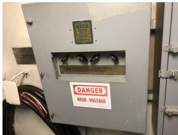
Figure 3: ASCO Transfer Switch (Image © 2022 Norbert Doerry – Licensed via CC BY 4.0)
