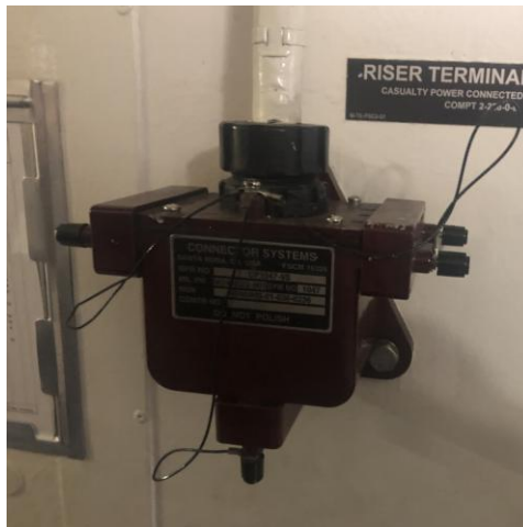
Figure 6: Casualty Power System Riser Terminal (Photo © 2024 Norbert Doerry, Licensed via CC BY 4.0)
