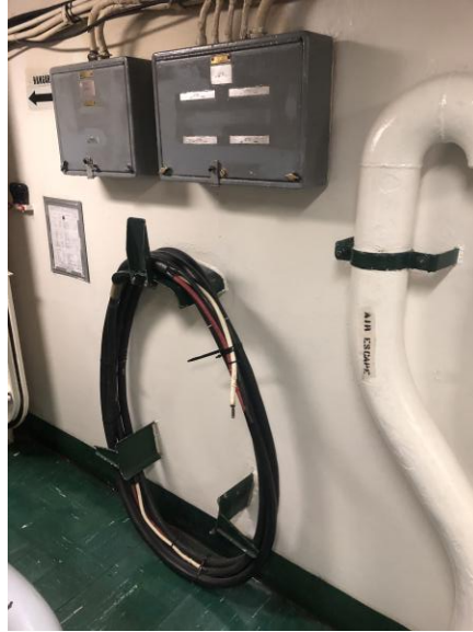
Figure 7: Casualty Power System Cable (old style termination) (Photo © 2022 Norbert Doerry, Licensed via CC BY 4.0)
